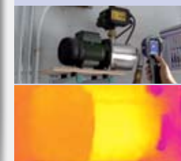
Inspection of this water pump shows no problem. The infrared image verifies that there is water in the pump cylinder and there is no danger of overheating the pump.
